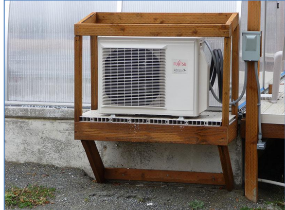
Ductless mini-split heat pump outdoor unit
