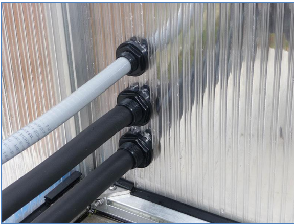
Glazing penetrations for refrigerant lines and power
